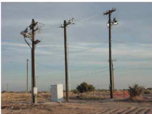
Point of Common Coupling Equipment
